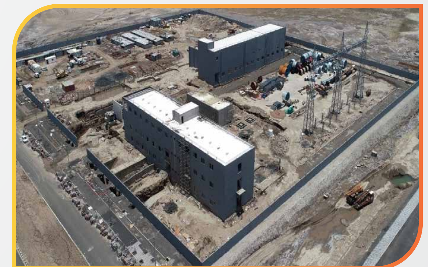
Torrent Power 440 KW Sub Station Operational
