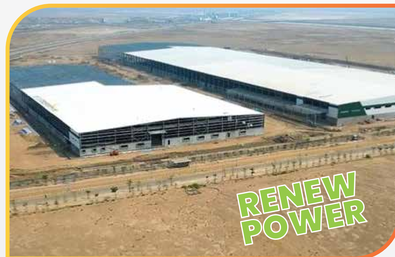
Renew Solar Pannel Plant Worth Rs. 1200 Carore in 100 Acre Area Operational Soon....
