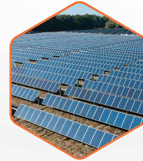
World's Biggest 5000 MW Solar Park in 110 Sq. Km.
